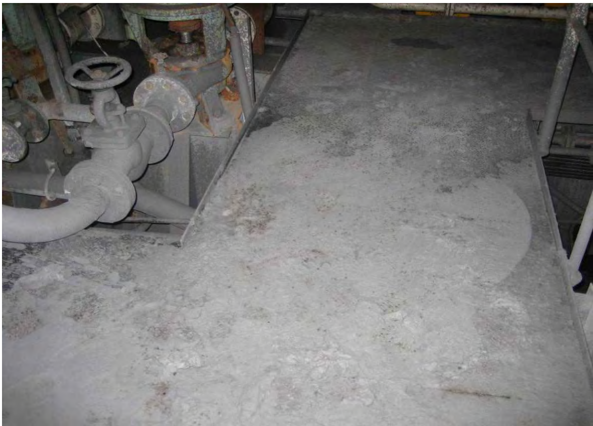
Figure 17 - Slurry on the Access Walkway in the Engine Room
