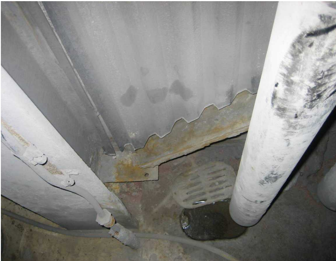
Figure 21 - Blocked Deck Drain - Port Side Deck
