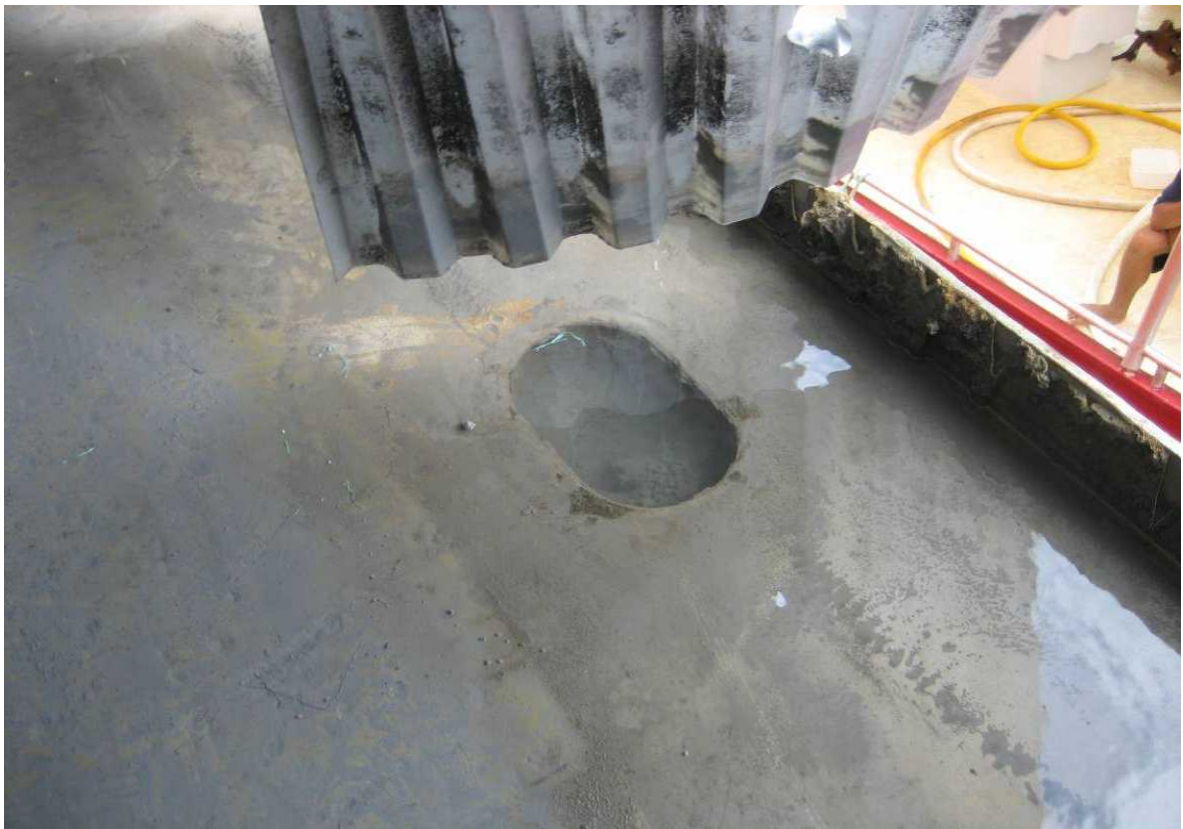
Figure 19 - Blocked Deck Drain - Port Side Deck
