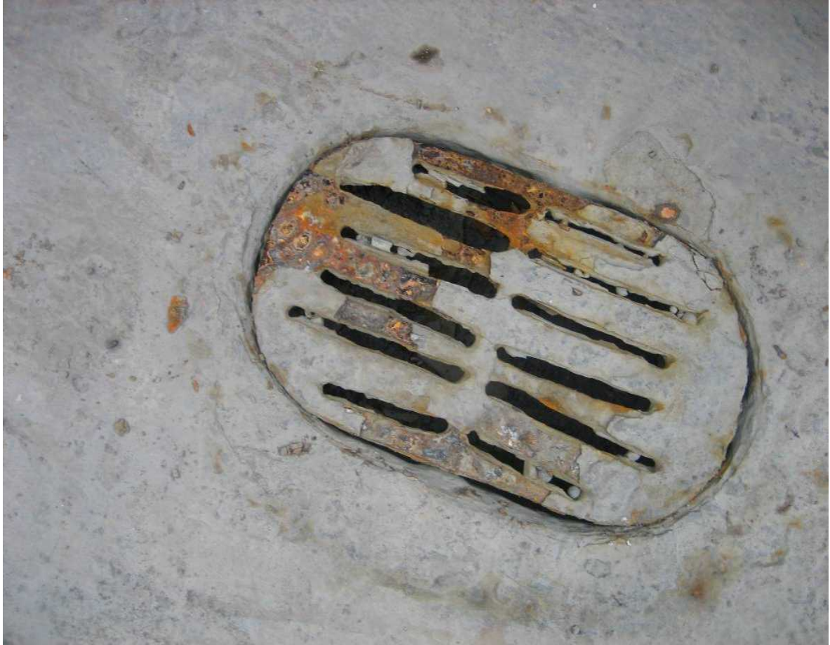
Figure 18 - Blocked Deck Drain - Starboard Deck
