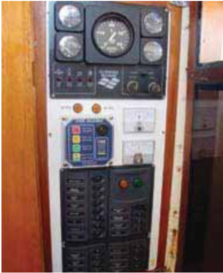
A DC circuit breaker panel on a small commercial vessel. Fire alarm, warning lights, engine instruments, voltmeter and ammeter are also incorporated. A separate panel exists for the AC system.
