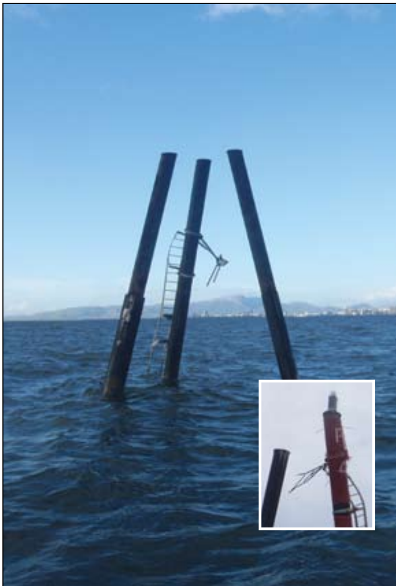
Above: Townsville sea channel leads suffered considerable damage during STC Yasi Inset: The leads have been temporarily restored to allow night shipping through the channel.
