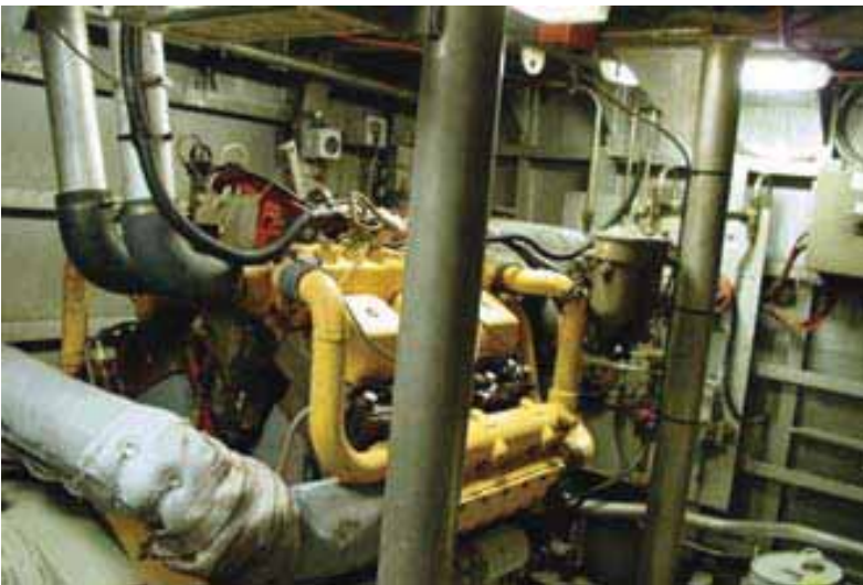
An auxiliary diesel engine such as this one may also be present in the engine room. It drives a 240 generator powering refrigeration, air conditioning, lighting and other appliances common on today's commercial ships. Care must be taken when working in a machinery space, as hot surfaces, moving machinery and a great deal of noise make this a hazardous environment at sea. Always wear appropriate PPE.
