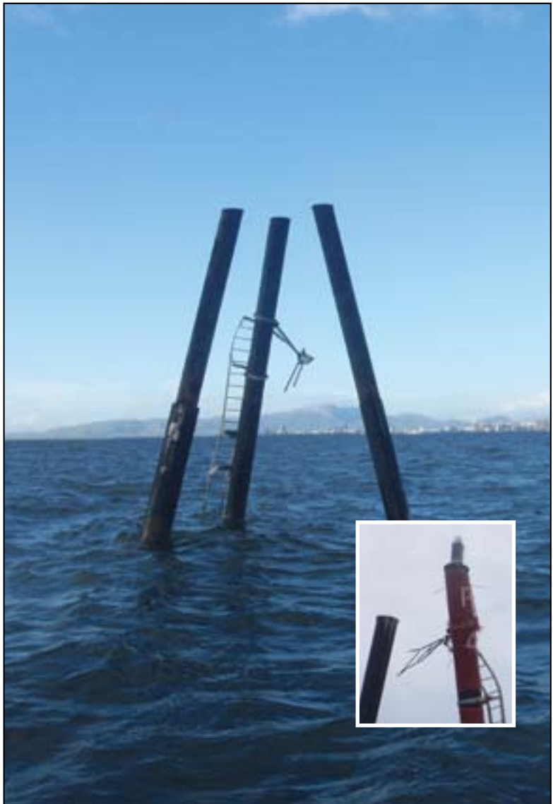
Above: Townsville sea channel leads suffered considerable damage during STC Yasi Inset: The leads have been temporarily restored to allow night shipping through the channel.
