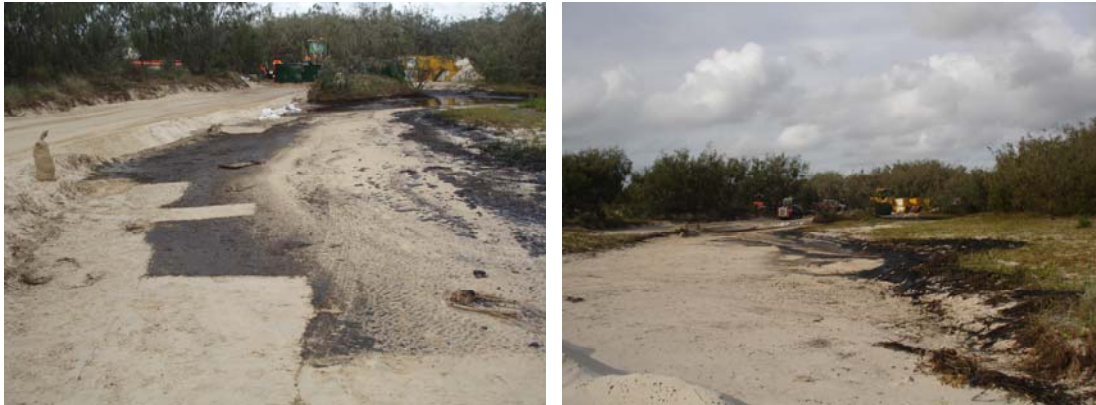
Figure 18: Oiling near the mouth of Eagers Creek. This needs to be removed ASAP using standard manual methods (shovels etc) to prevent potential re-pollution of the wetland (Moreton Is. East Coast 18/3/09).
